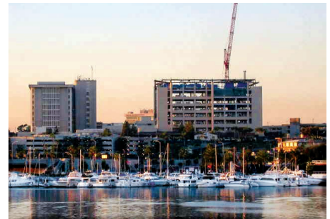
Top to bottom: Starting, November 2001; footprint of the building and the springs it sits on; harbor view of nearly completed project
